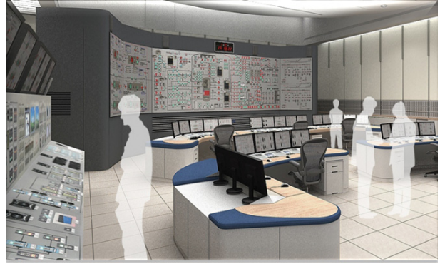
Figure 1. APR1400 main control room
